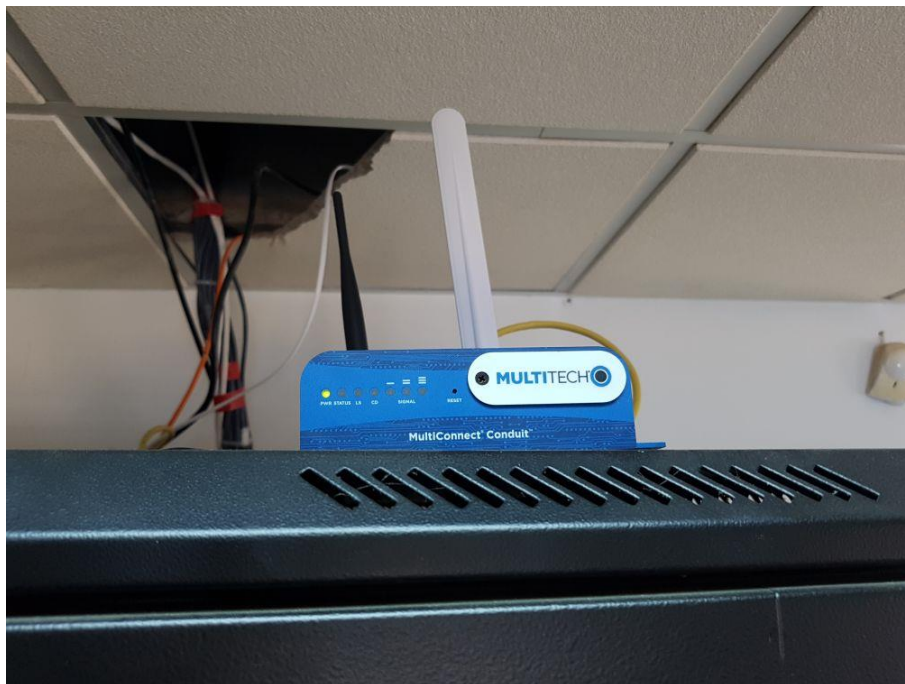
Figure 17: Installed gateway (ELDIA)
