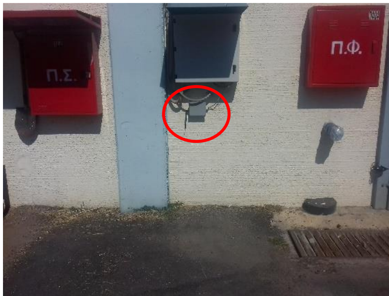
Figure 15: Installed gateway (KLEEMANN)
