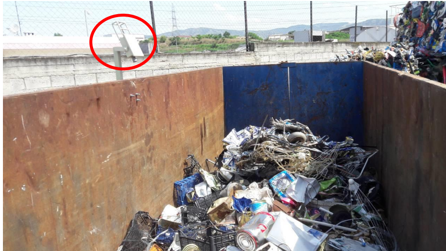
Figure 18:Outdoor fill-level sensor installed (ELDIA)
