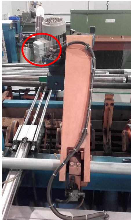
Figure 8: Vibration Sensor installed on Bossi Motor
